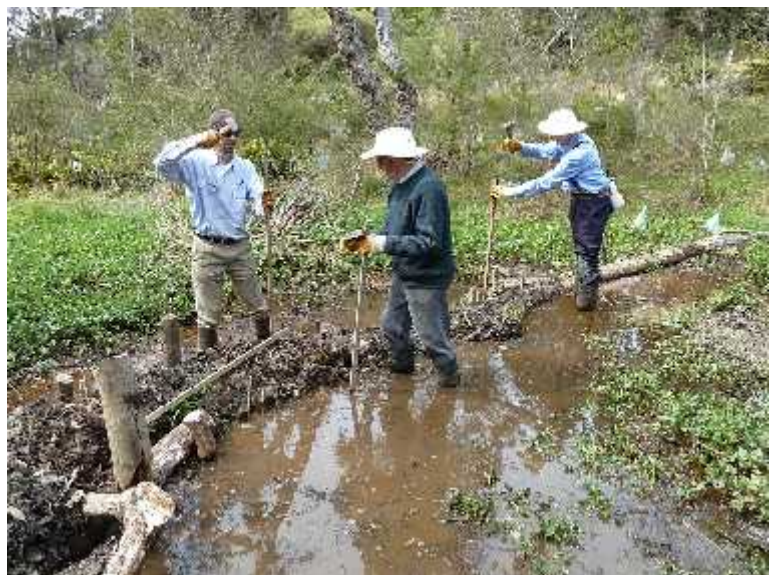
Photo 4. Building a detention cell from woody debris. The carpet of Creeping Buttercup seen here exploded when we started removing the willows and opened the ground up to light. However it served the useful purpose of protecting the surface while our plantings became established and we found later that it was suppressed by the raised water table.
