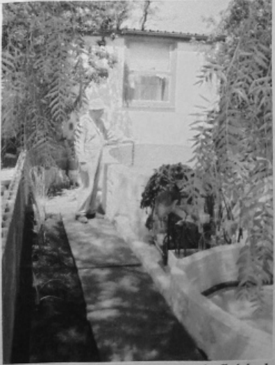
The storage pond, settling pond, low pond and bog garden. Nearly finished.
